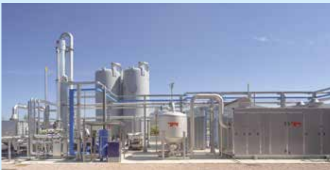
Biogas upgrading plant of Snam 4 Environment (capital 100% Snam S.p.A.), 3-stage HPSM membrane system for the production of Biomethane
